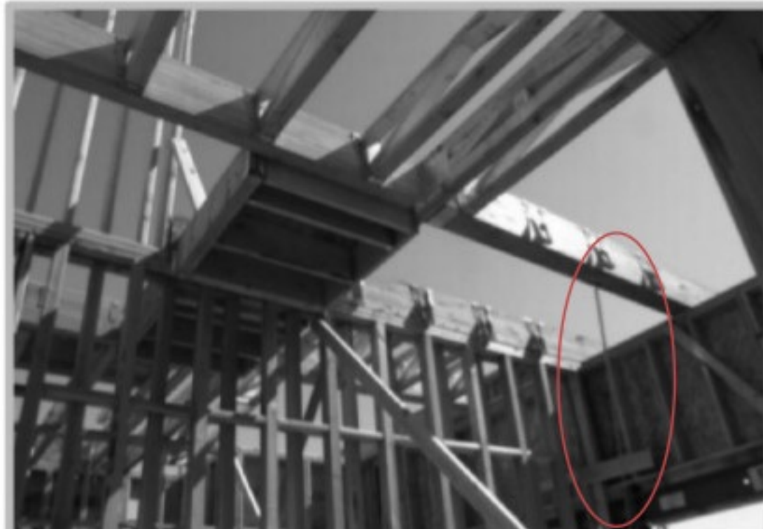
Photo of incident scene showing the opening the worker fell through while installing floor trusses.
